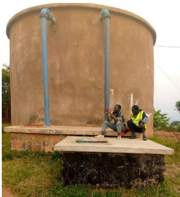
Figure 12: Existing water tank in Kibeho Sector, Nyaruguru District
