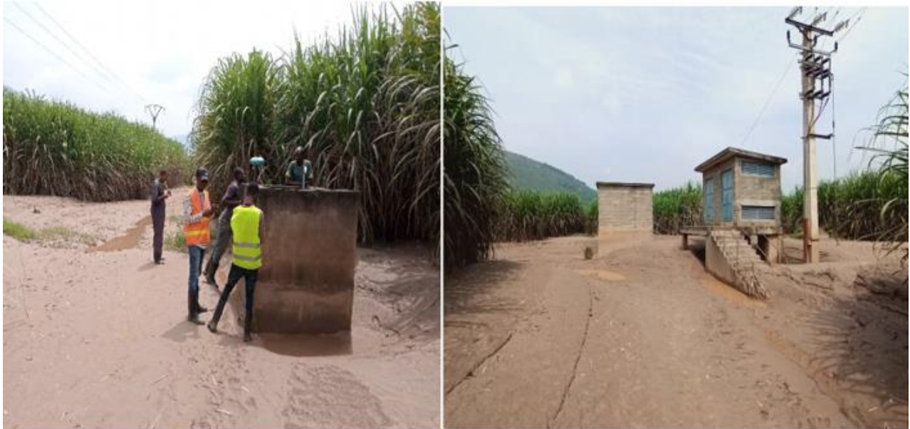
Figure: One of the borehole top structure(left) and raw water collector chamber with its transformer(right) belonging to the well field for groundwater all located in Nyabarongo plain.
